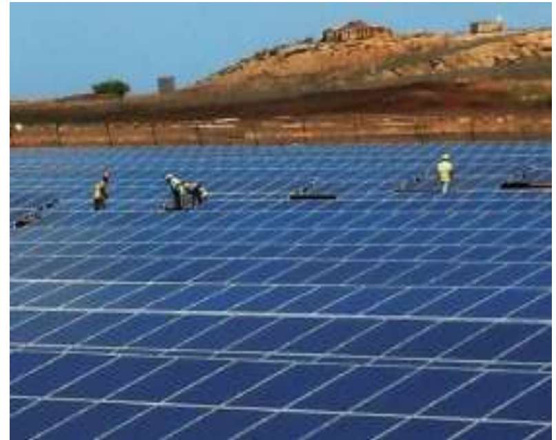
5 MW Solar PV, in Praia, Cape Verde Commissioned November 2, 2010
